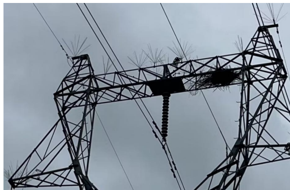
Figure 5 and 6. Oriental storks on power tower.
