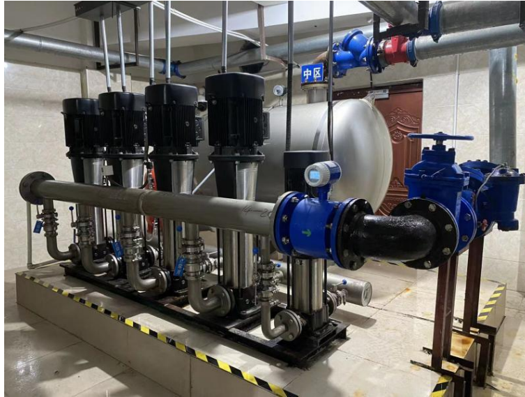
Pump station in Steel plant. Photo source: YAO Fulai
