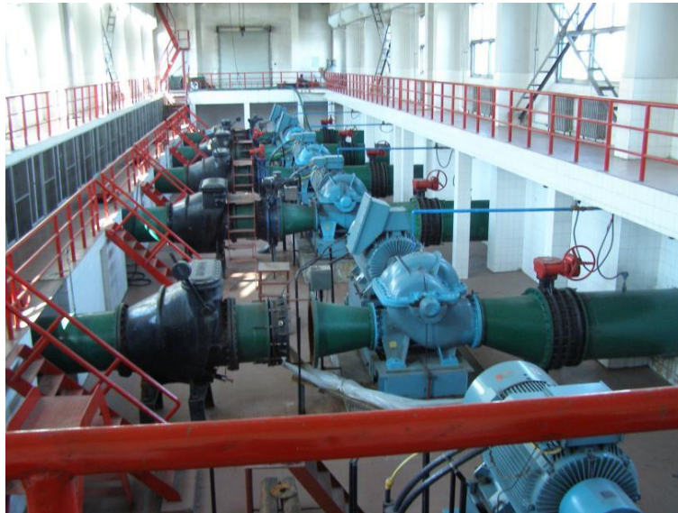
Pump station in water plant. Photo source: YAO Fulai
